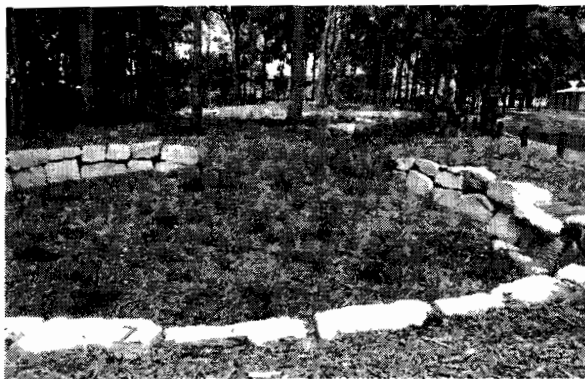
A swale and bio-retention basin will treat stormwater. Source: Water by Design
